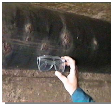
Poor surface preparation and continuing moisture produced these corrosion cells.
