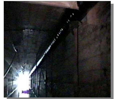
The final view from within. The recoated pipe in place and awaiting deliveries.
