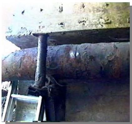
The destructive result of coating loss, environmental exposure and time.
