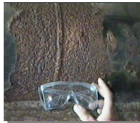
Precise pit depth readings were taken to help assess extent of damage.
