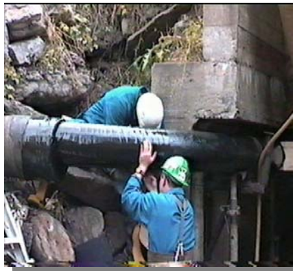
Casing end was first sealed then both pipes were wrapped with KemaSeries60.
